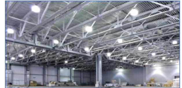
AEP Ohio Adv. Lighting Controls
